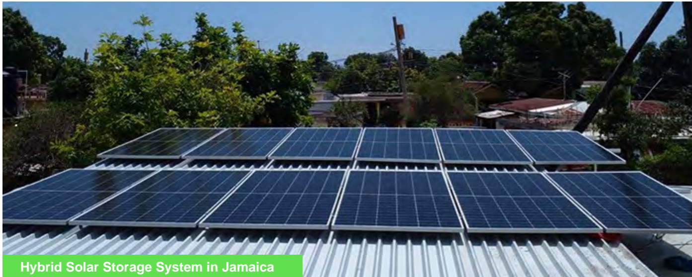
Jamaica household solar storage project
